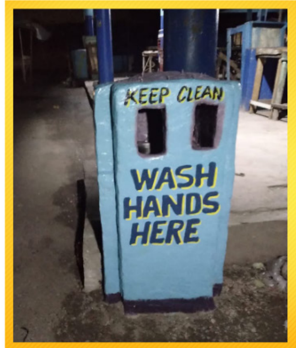
Figure 2: Newly installed handwashing station at the Old Harbour Bay Fishing Village
